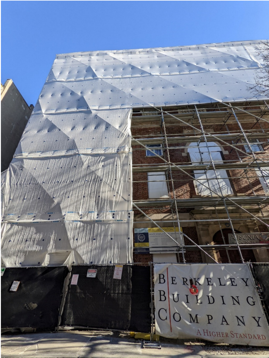
In the North End, CPA funds supported the adaptive reuse of the existing Knights of Columbus headquarters to create 23 affordable apartments for seniors, including three units reserved for seniors experiencing homelessness. This CPA project also developed meeting space for the North End community and acquired a new space for the Knights of Columbus. Source: JM Goldson
